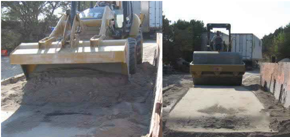
Figure D-2. Grid positioned over compacted base and covered. Cover soil/aggregate is uniformly spread and compacted using field-scale equipment and procedures.
