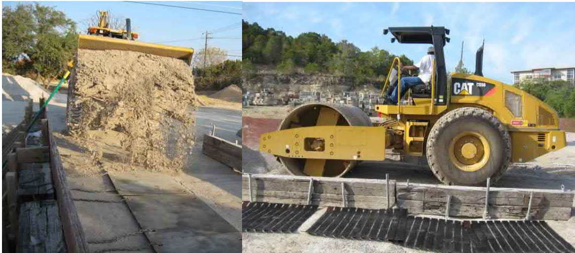
Figure D-1. Lifting Plates positioned between ties and covered with first lift of compacted soil/aggregate.
